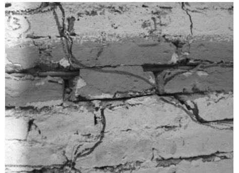
图7 嵌入钢筋外露 Fig. 7 Exposure of the embedded steel bars
