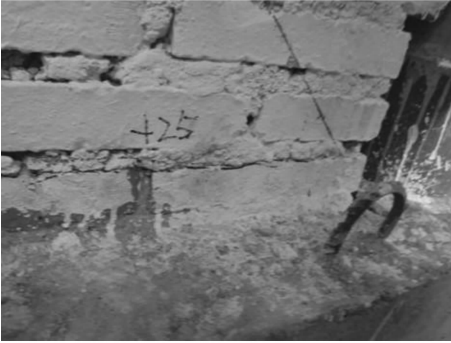
图4 砌体墙水平裂缝发展 Fig. 4 Progress of horizontal cracks in the masonry wall
