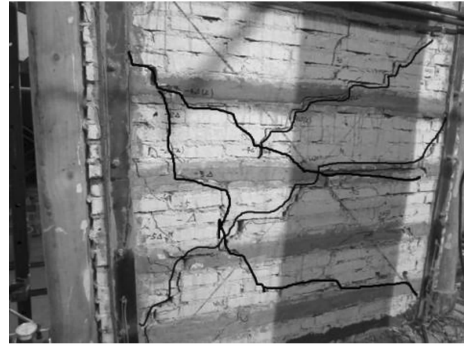
图6 试件 KJ-2 破坏形态 Fig. 6 Failure mode of specimen KJ-2
