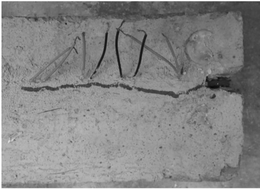
图 14 试件 T4.5-L450-300 的混凝土-树脂界面裂缝 Fig. 14 Crack at epoxy-concrete interface of specimen T4.5-L450-300
