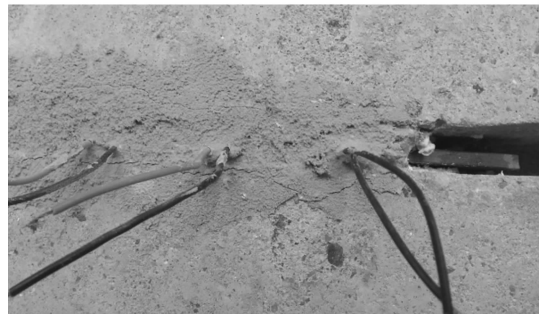
图 13 试件 T4.5-L450-150 槽两侧黏结界面的裂缝 Fig. 13 Cracks at interface on both sides of groove of specimen T4.5-L450-150
