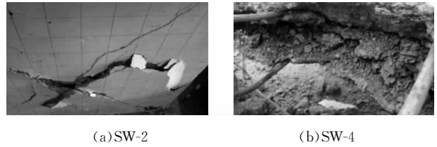
图7 混凝土保护层剥落和内部混凝土分层的照片 Fig.7 Photographs of concrete crumbling and internal concrete layering after testing
