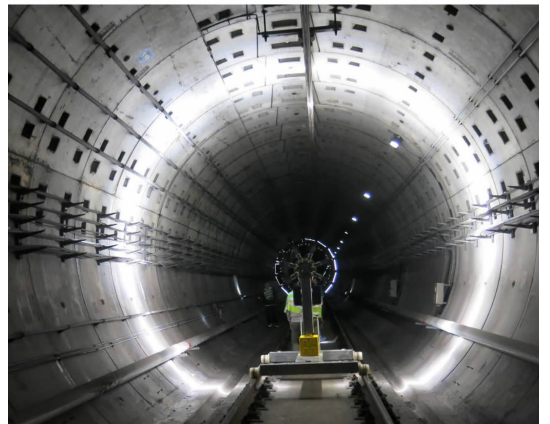
图 2 MTI-100 隧道病害检测 Fig. 2 Tunnel disease detection with MTI-100
