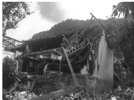
(a)架倒墙塌
