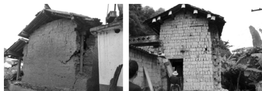
(c)外墙局部坍塌
