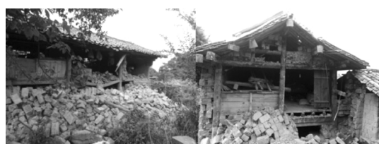
(b)墙倒架不塌
