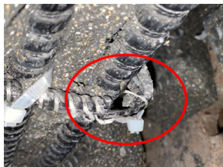
图6 箍筋的弯曲处断裂 Fig.6 Broken at the bend of stirrup
